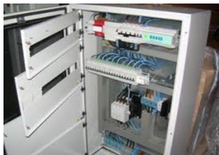
Imm.128: Electric station
