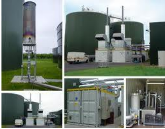
Imm.135: Biogas plant
